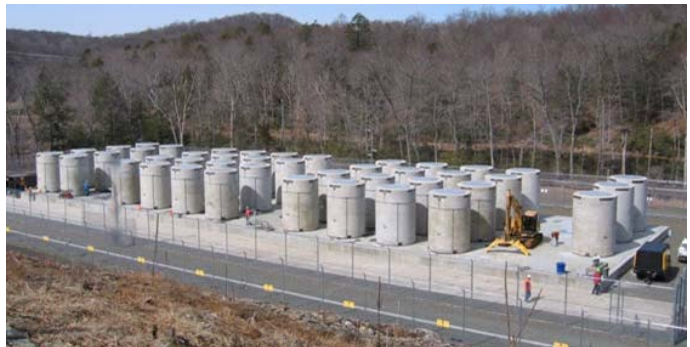
Typical ISFSI (photo by permission: NAC International)
