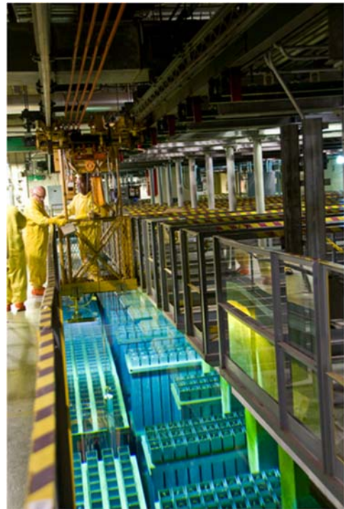
Figure 3. Spent Nuclear Fuel Storage in the Vertical Tube Storage area at the L Basin (from Hixson 2015).
