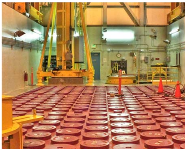
Figure 4. Inside the Fort St. Vrain SNF Dry Storage Facility (CH2M-WG Idaho, LLC 2012).
